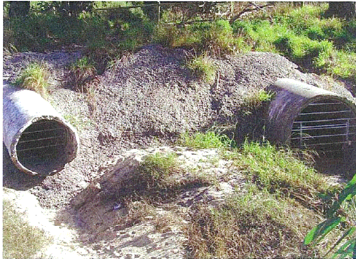
Photo 1 Catchment 1 675mm Outfall and Catchment 2 1050mm Outfall
