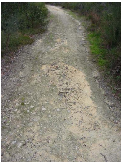
Plate 5.1 Minor erosion of limestone path
