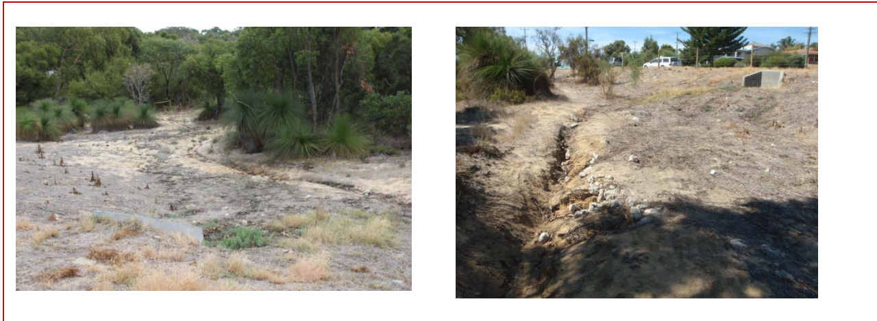
Figure 8: Culvert near Charles Riley Road and Associated Erosion
