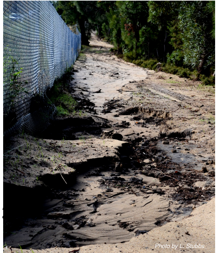
Uncontrolled erosion on road reserve adjoining a conservation reserve Paganoni Swamp.
