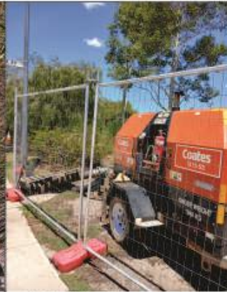
16/4/26 Pumping out swale along Mayfield Drv, Brabham
